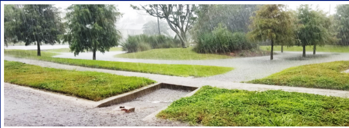
Innovative Above Ground Detention Area in Retrofitted New Orleans Stormwater Lot; source: Louisiana.gov
